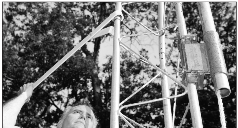
Figure 3—During tower assembly, you'll occasionally run into situations where some alignment adjustments are needed to get the third leg to insert. The Leg Aliner can provide the necessary force.
